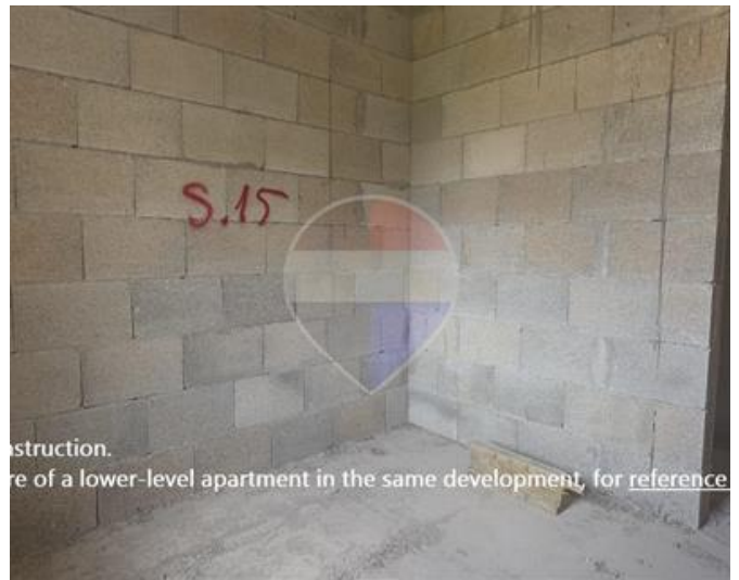
...ruction. ...of a lower-level apartment in the same development, for reference only .
